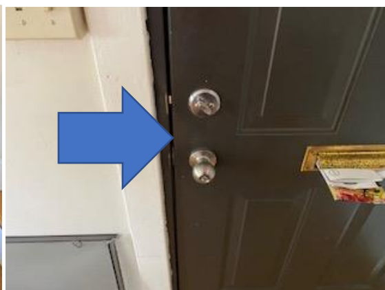
Door Hardware - Inside
