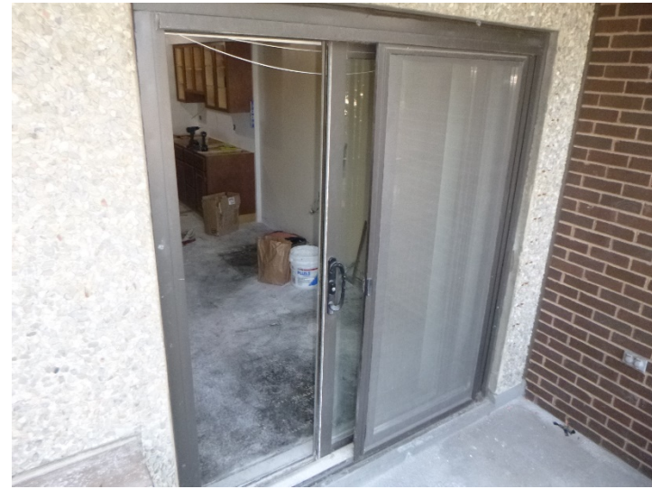
Typical sliding glass dwelling unit balcony/patio door.
