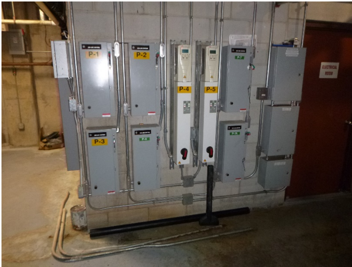
View of the variable frequency drives (VFDs) that govern two base-mounted 5-horsepower circulator pumps.
