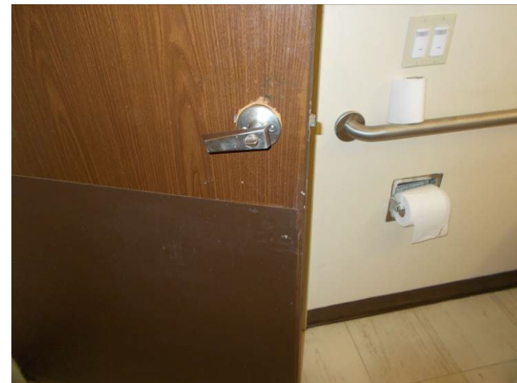
The locking hardware on the common restroom requires pinching and turning which is non-compliant.
