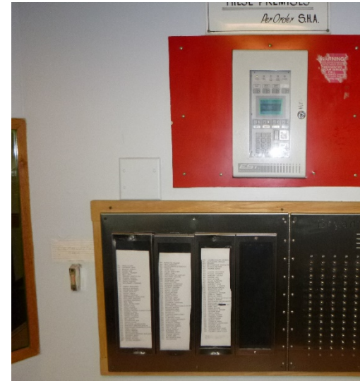
The EST fire alarm control annunciator panel (bottom) located in the entrance.
