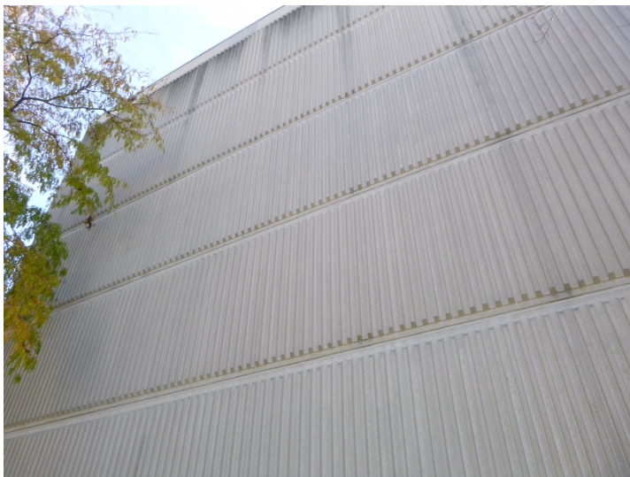
Typical condition of the precast concrete panels at an end wall. Note: Staining at upper section of the wall.
