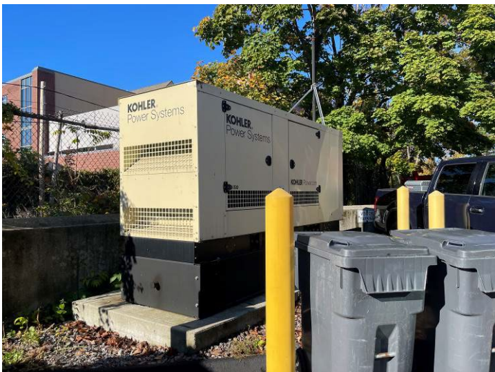
View of the Kohler 100 kW stand-by generator which was installed in 2016.
