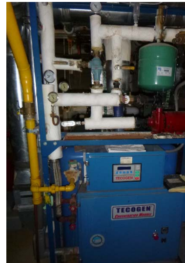
The Tecogen cogeneration system that produces domestic hot water and supplemental electricity for the building.
