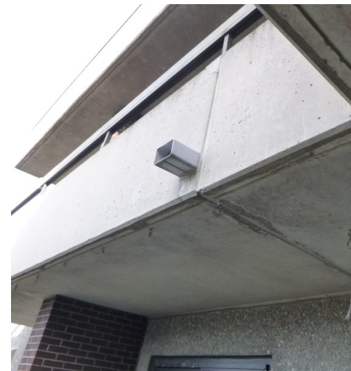
No significant cracking/deterioration was observed on the underside of balconies from available
