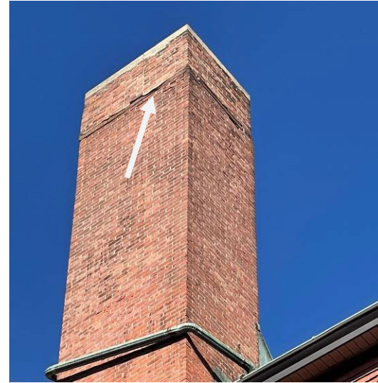
View of the chimney, note the mortar loss at the upper courses of brick.
