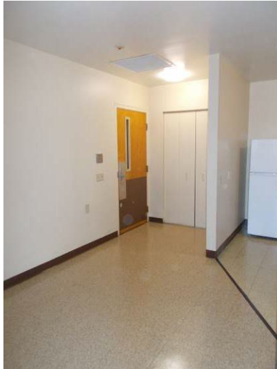
View of typical unit living area finishes. Note locking hardware on the entry door requires pinching and turning which is non-compliant.
