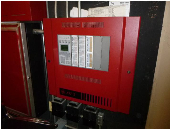
The EST fire alarm control panel.
