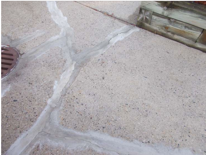
Pedestrian access provided by concrete walkways, previous cracking and repair efforts observed.
