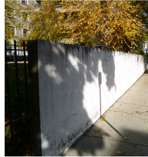
The concrete retaining wall along a section of the city-owned public sidewalk.
