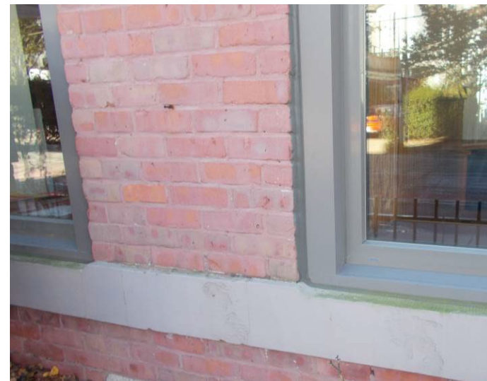
Vinyl framed windows are less than ten years old. The caulking appears to still be pliable.
