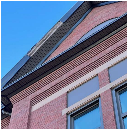
Area of rake board trim cladding missing at the front façade.
