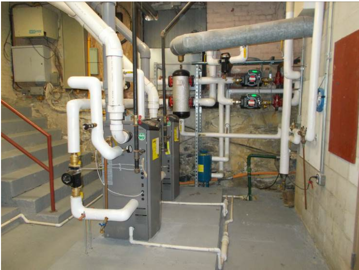
View of the Lochinvar heating boilers and circulation pumps.
