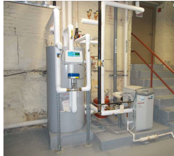
View of the Lochinvar domestic hot water boiler, storage tank, and Heat-Timer ETV Platinum Plus control valve.
