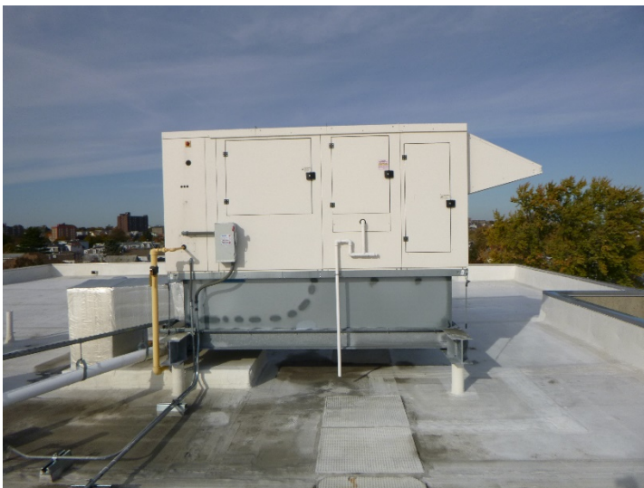
One of three recently replaced Reznor roof mounted makeup air units (MAUs).
