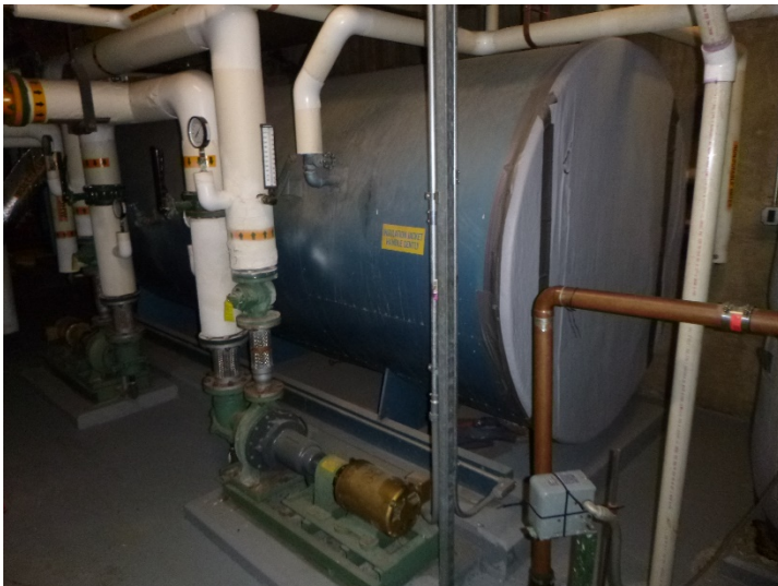
View of the domestic hot water storage tank.
