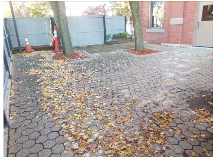
View of the concrete pavers at the patio off of the first-floor lounge.
