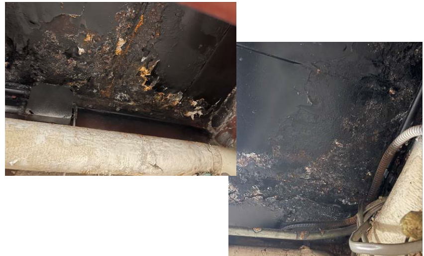
Area below vestibule with deterioration of the metal pan flooring system.
