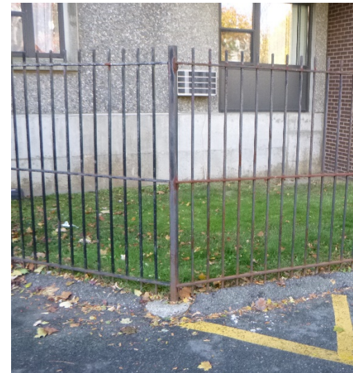
The painted metal picket fencing exhibits surface rust.
