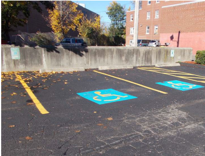
View of the accessible parking space which lacks an access aisle.
