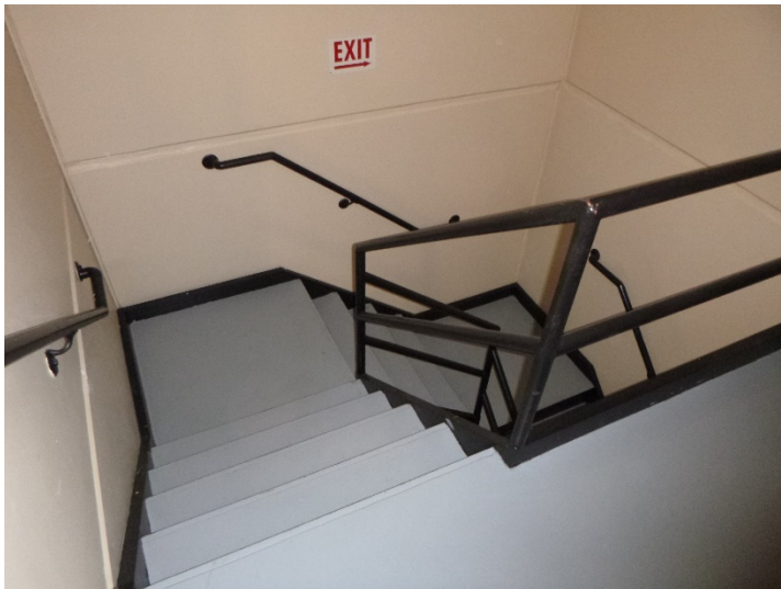
Typical egress stairwell finishes and condition. Note: stairwell railings do not meet current accessibility or safety standards.
