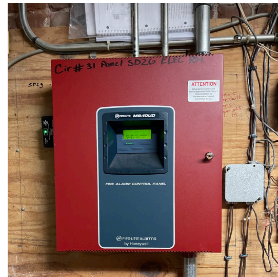
View of the FireLite MS-10UD fire alarm panel which was installed in 2015.
