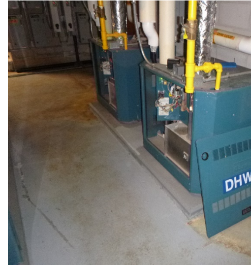
The domestic hot water backup boilers are Burnham boilers.
