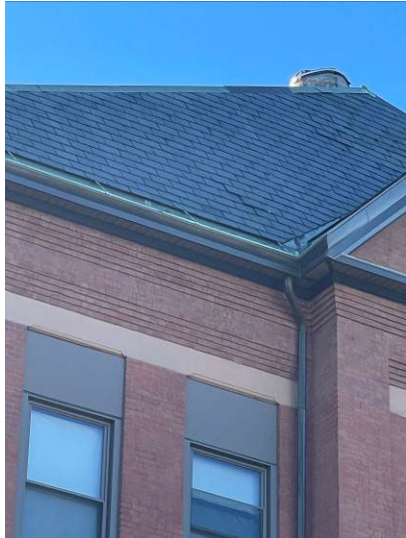
Lifting shingles at the front of the building will be repaired in 2022.
