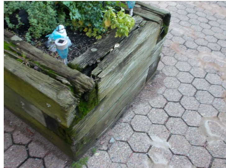
Flower box at the direct entry unit with wood tie retaining walls; note the deterioration.
