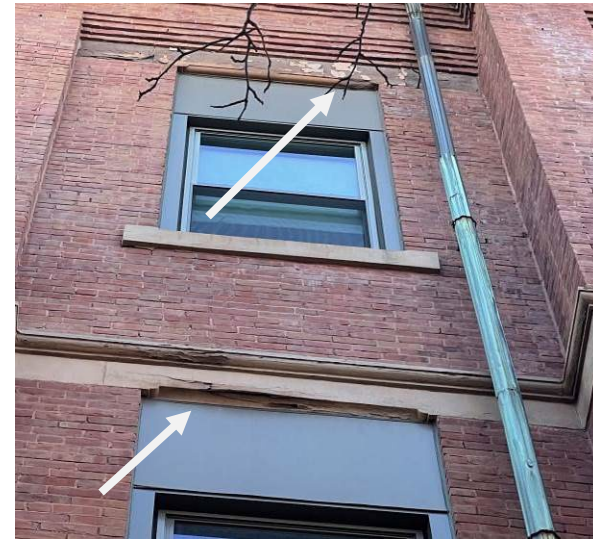
Additional areas of concrete banding damage.
