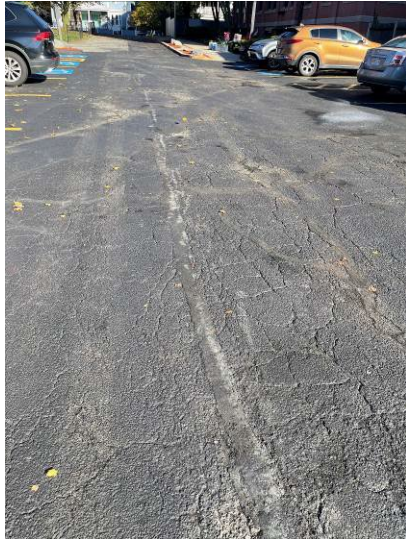
View of the asphalt paved parking area, note extensive cracking and deterioration observed.
