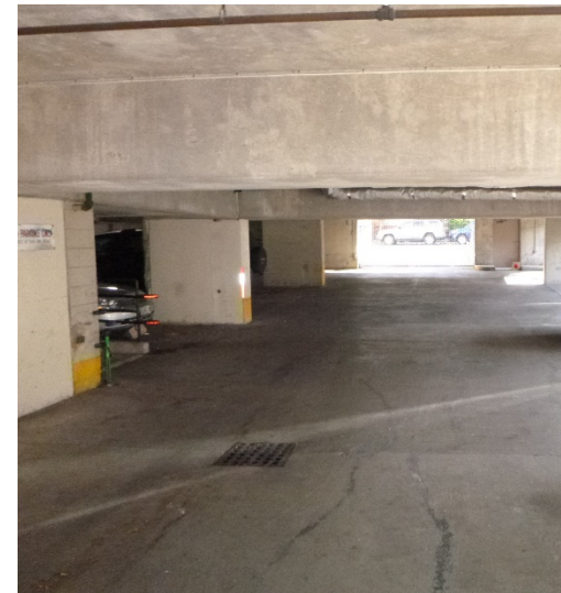
View of the parking garage located under the building. Note: faded striping and evidence
