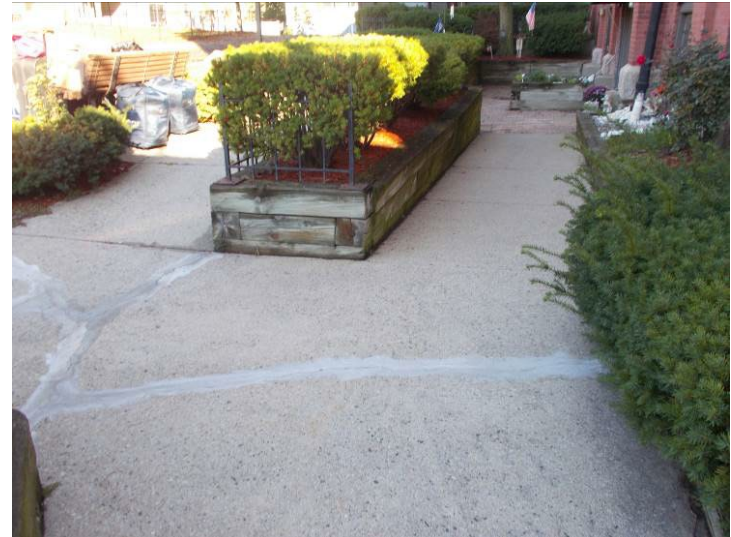
View of the concrete ramp to the lower-level units lacking handrails.
