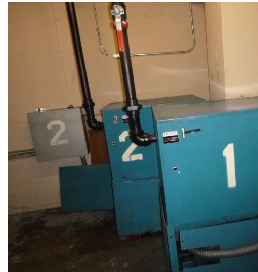
View of the two hydraulic elevators.
