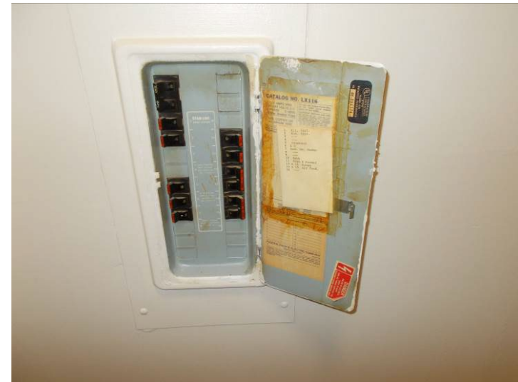
Units have Federal Pacific Electric (FPE) 'Stab-Lok' circuit breaker panels.
