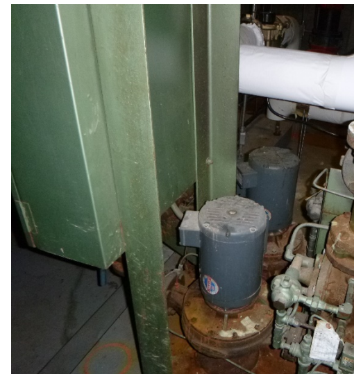
The original cold water booster pump skid with two pumps and control
