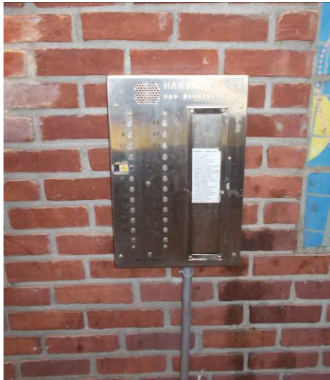
Visitor access is controlled by a vandal-resistant stainless-steel door buzzer/intercom panel at the entry lobby.
