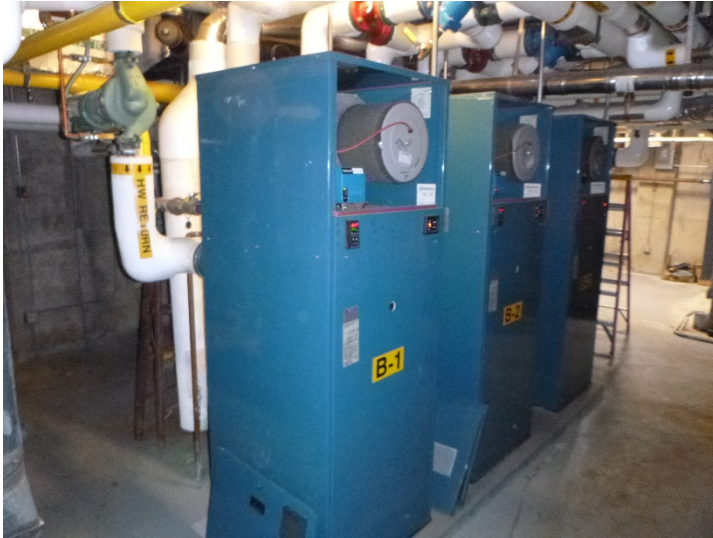
Three Thermal Solution Evolution, modulating, gas-fired boilers produce hydronic heat for the building. Each boiler has a rated input capacity of 1,500-MBH.
